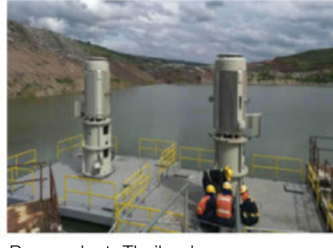
Power plant, Thailand
