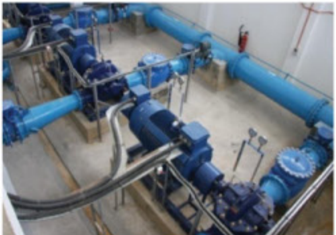
Water plant, Malaysia
